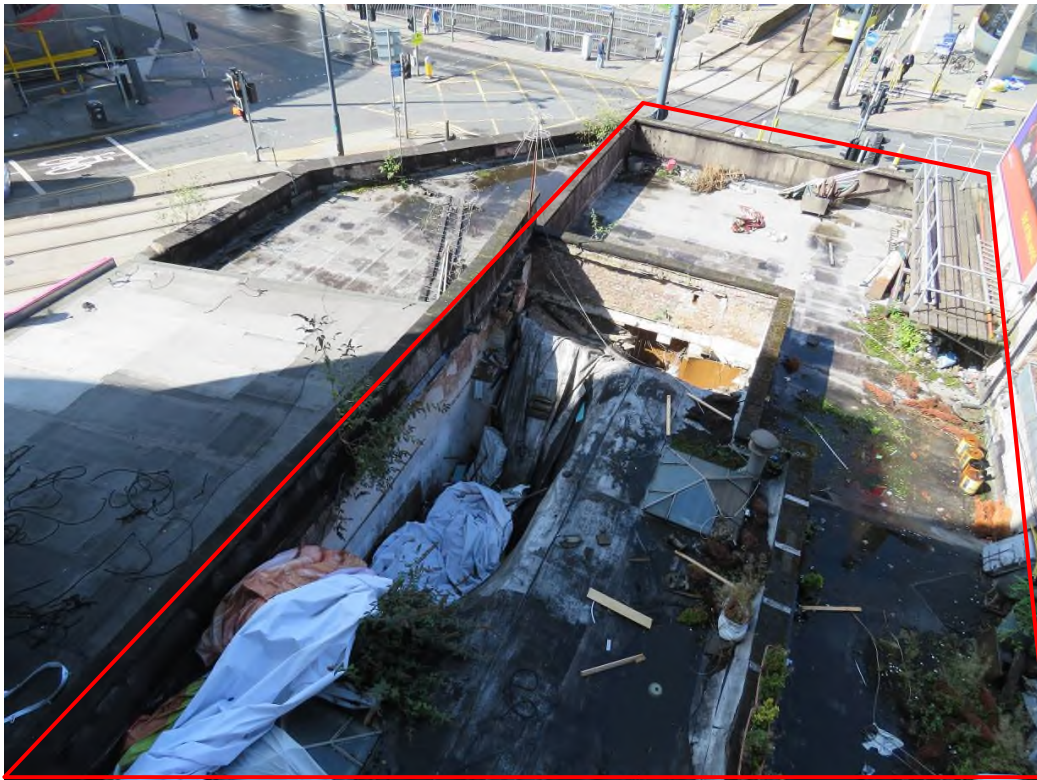
The collapsed rear of 30 - 32 Shudehill
